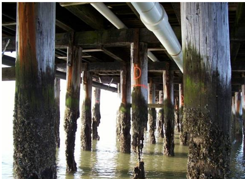
Figure 6. Effect of marine borers on wood structures (SAWPA).
